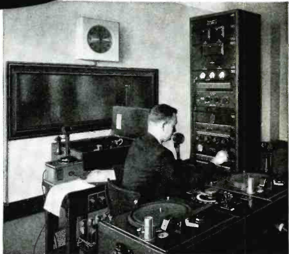
Control room at WHAT, showing 9A Speech Input Equipment with Moving Coil Microphone and Western Electric Reproducer Set
